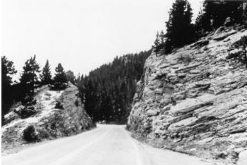
Figure 3.16: Typical Roadway with Roadside Hazard Rating of 7: Clear zone less than or equal to 5 ft; side slope about 1V:2H or steeper, non-recoverable with high likelihood of severe injuries from roadside crash (Source: AASHTO, 2010).
